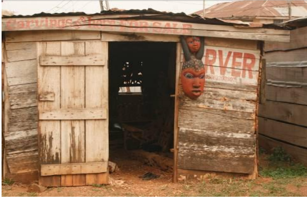
Plate VII: Dilapidated Shed. Source: Authors' Field Survey, 2013
