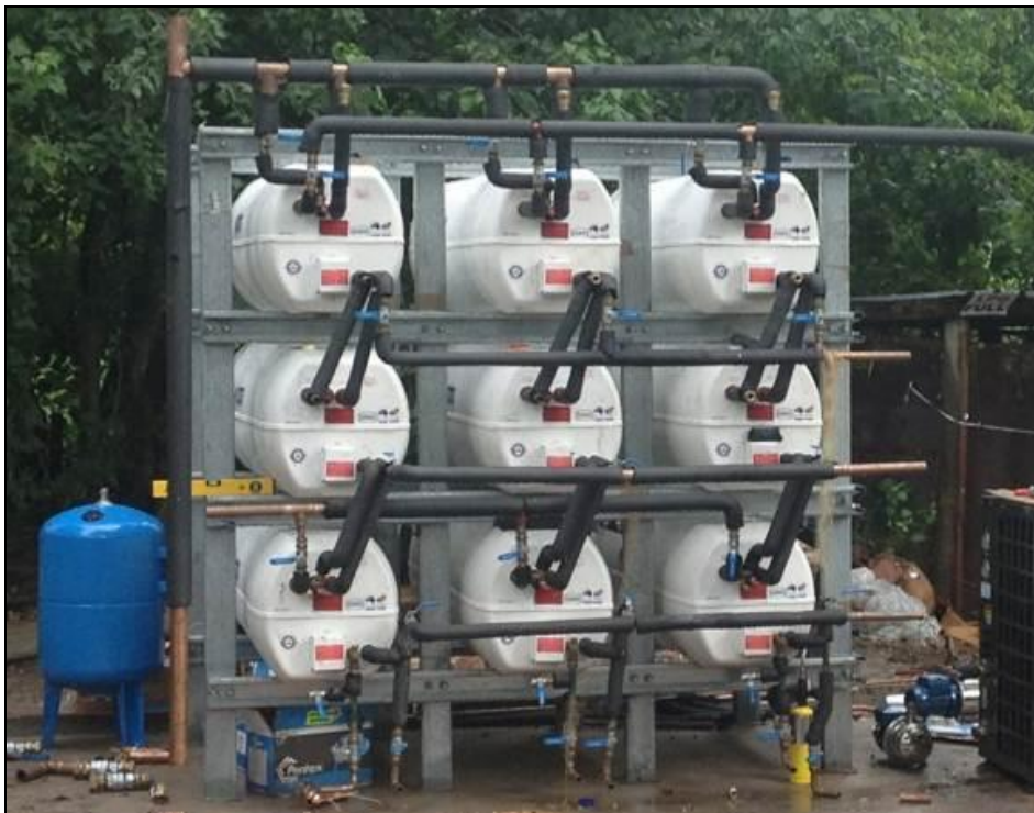
Figure 1: Photo taken during the installation of the bulk solar hot water system at Sandibe Okavango Safari Lodge in Botswana (photo courtesy of Jonathan Braack, andBeyond).
